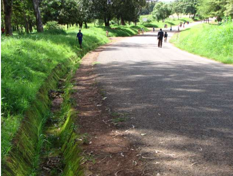
Brick-lined drain on longitudinal gradient of peri-urban section of the Ntchisi (school) road. Example of Satisfactory drainage
