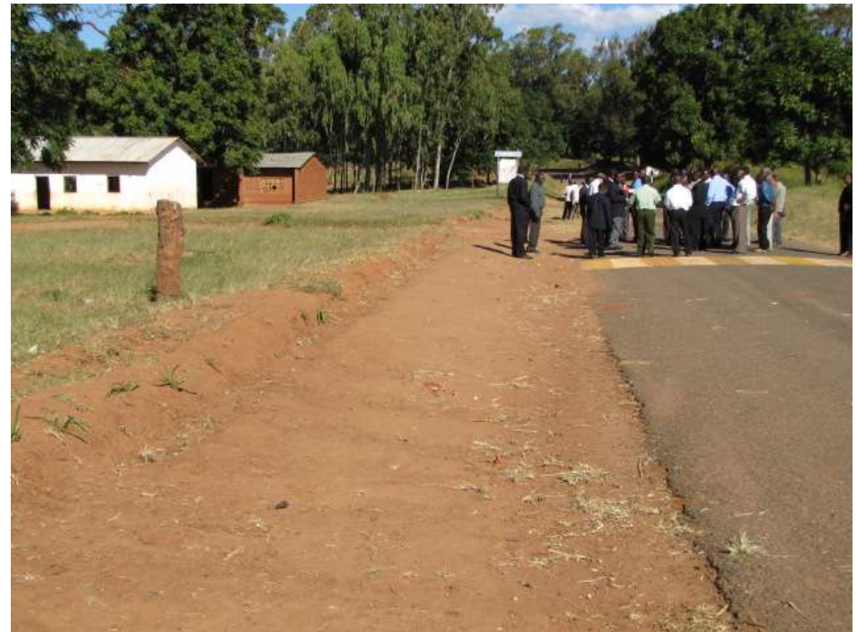
Poorly drained section of the Ntchisi (school) road. Example of poor drainage.
